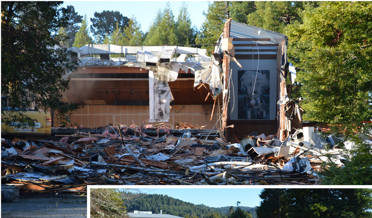
ABOVE AND RIGHT: Demolition of the old Life and Physical Science Buildings
